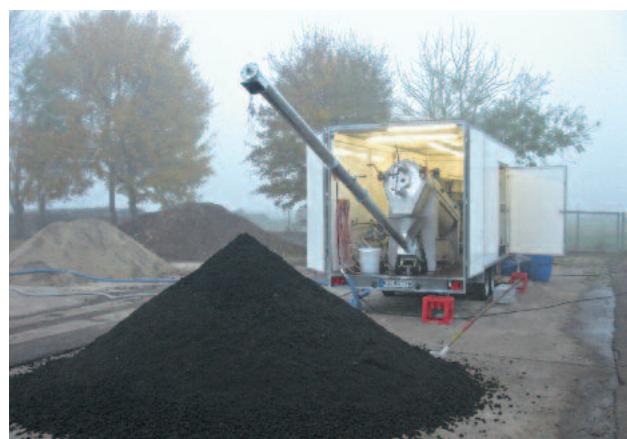
Contract dewatering with a trailer-mounted unit size 440
