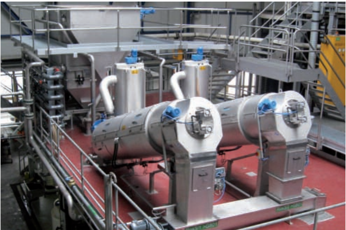
ROTAMAT® Screw Press RoS 3 units and HUBER Dissolved Air Flotation Plant HDF 5 with chemical treatment stage
