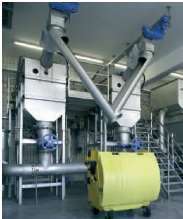
ROTAMAT ® Rotary Drum Fine Screen Ro 2 installed next to the HUBER Dissolved Air Flotation Plant HDF
