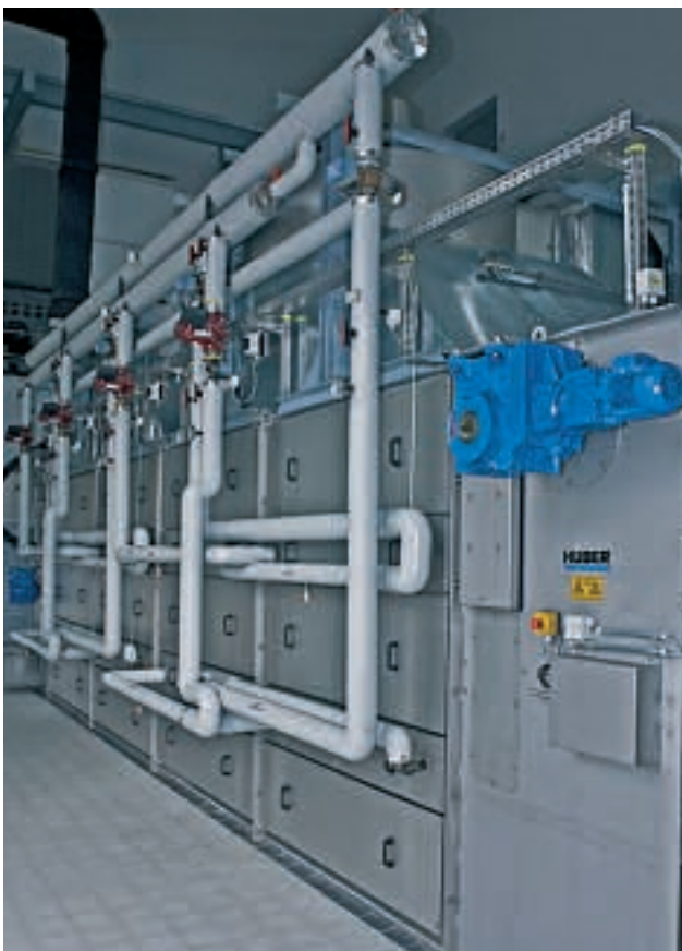
Biogas exhaust heat supply to a belt dryer
