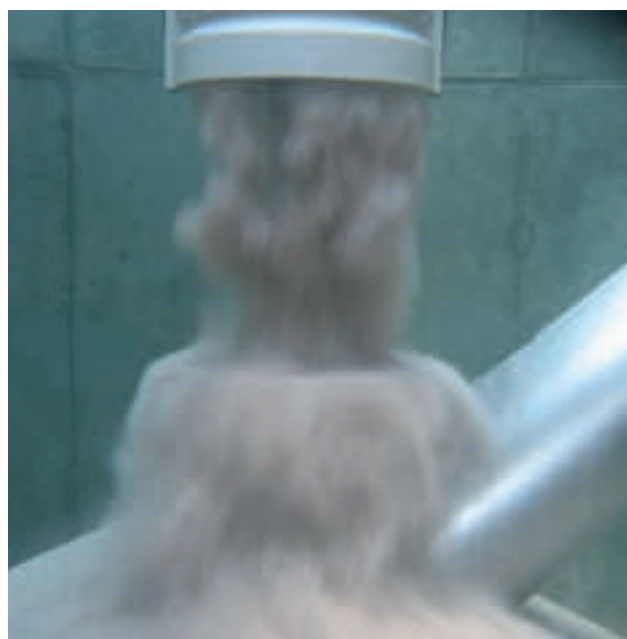
Crystal-clear effluent from the sandfilter
