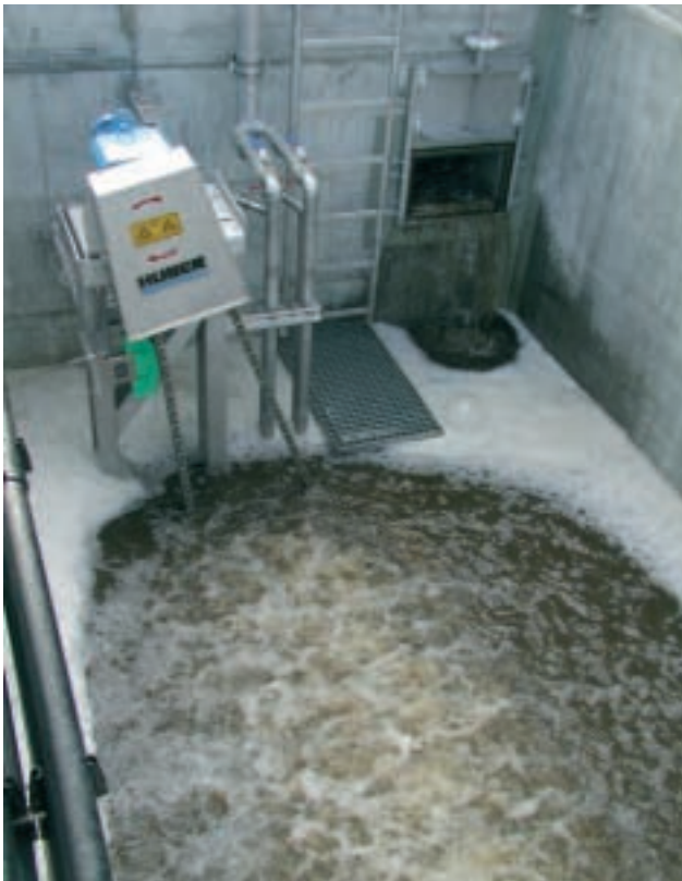
VRM® Membrane Filtration Plant
