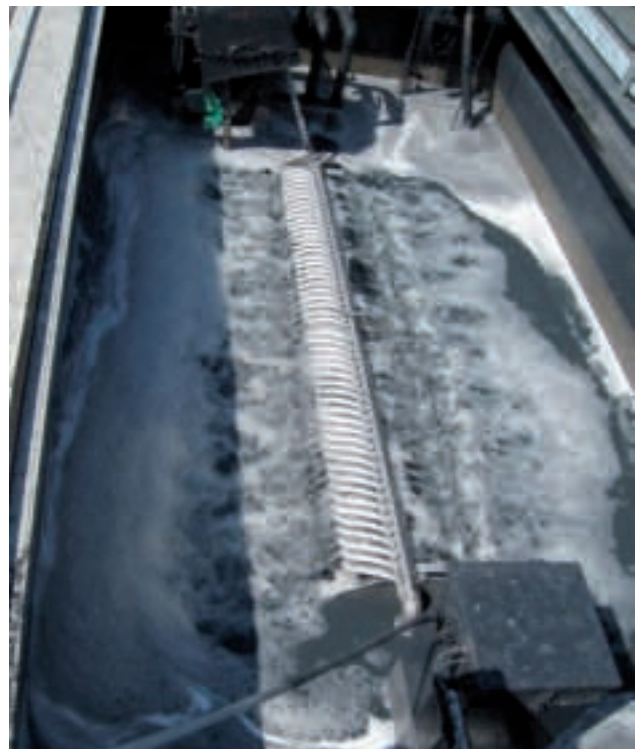
Scouring air introduction into VRM® plant
