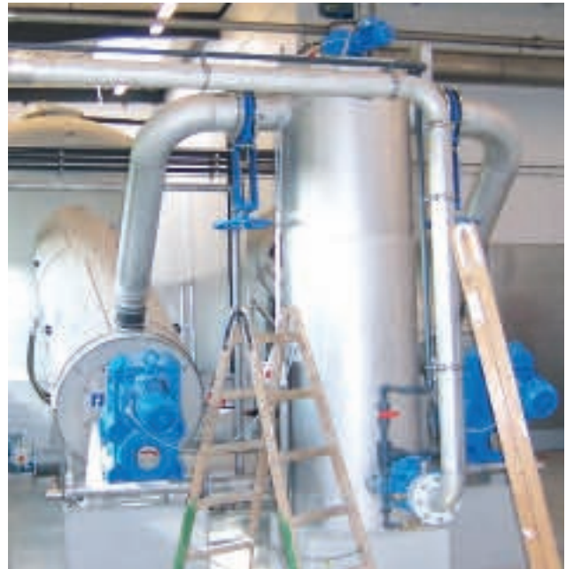
Flotate sludge dewatering with two ROTAMAT® Screw Press RoS 3/3 units with pipe reactor during installation
