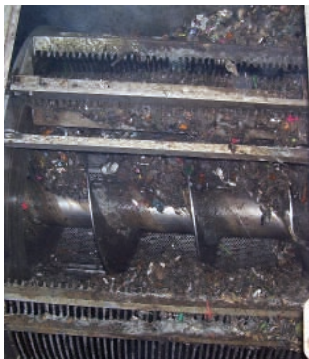
In the fine screening plant undissolved solids are removed from the organic suspension (approximately 5 – 15 % of the inflow)
