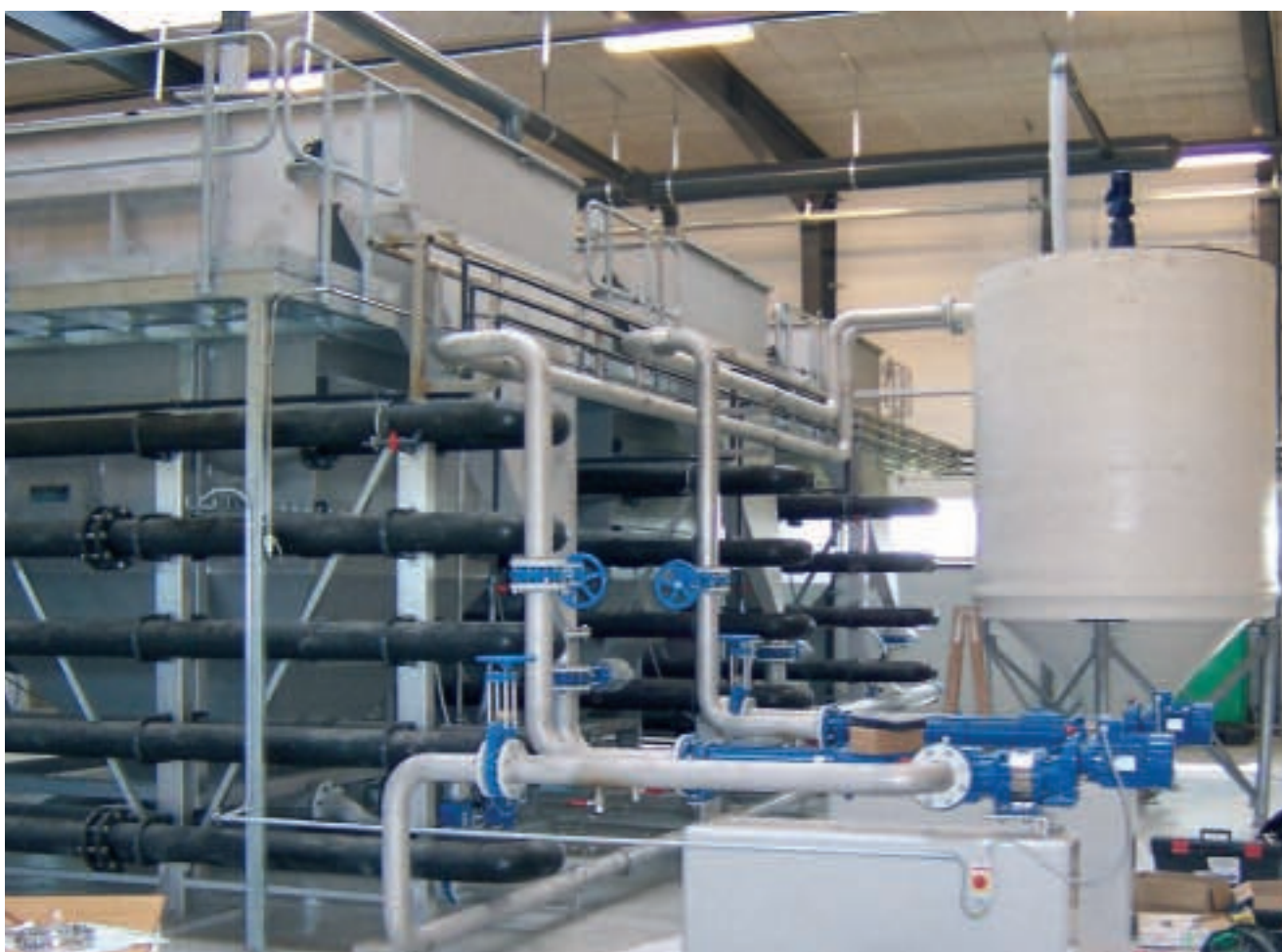
HUBER Dissolved Air Flotation Plant HDF 7 with chemical treatment stage and sludge tank
