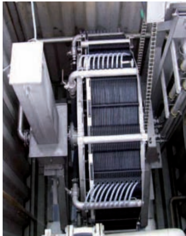
VRM® pilot plant: membrane biology with filtration chamber
