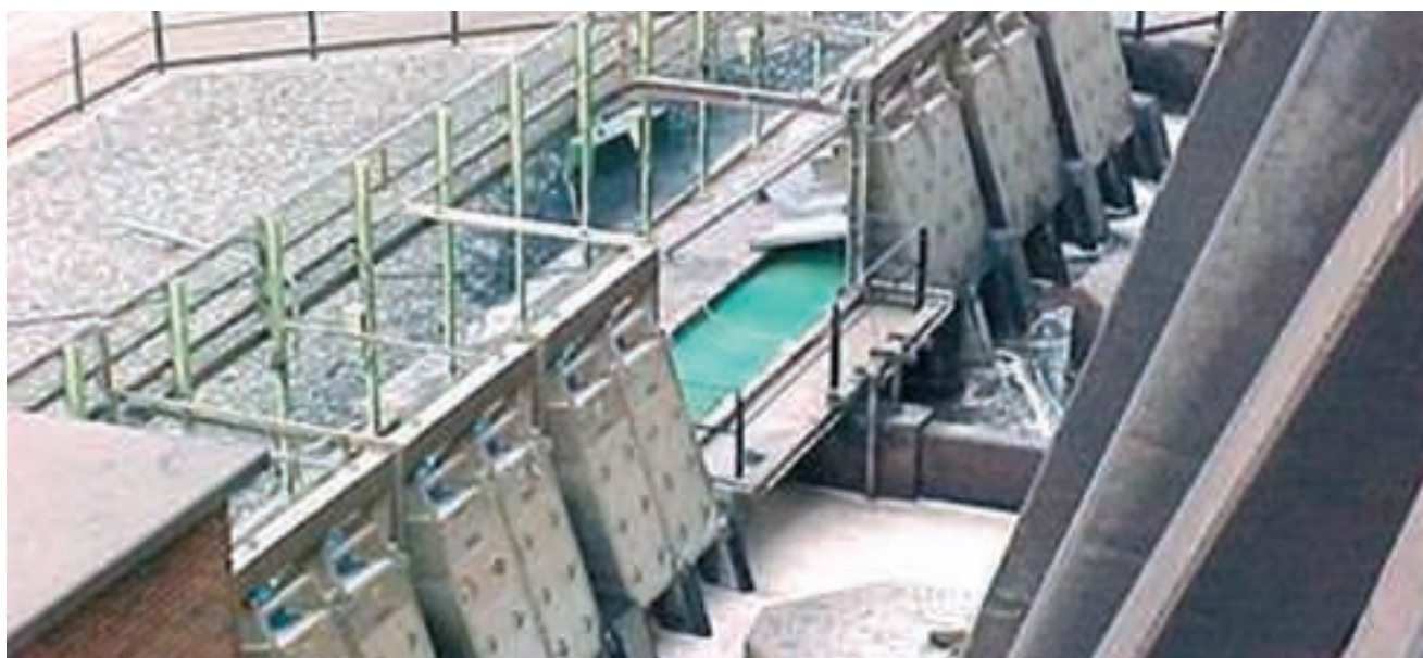
Seven HUBER STEP SCREEN® Vertical units installed in the inlet to the cooling tower
