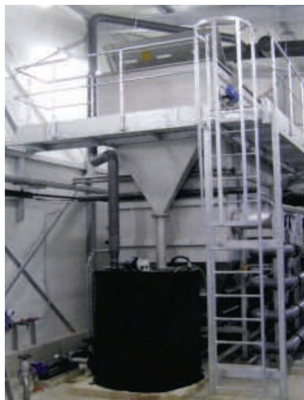
HUBER Dissolved Air Flotation Plant HDF 10 during start-up
