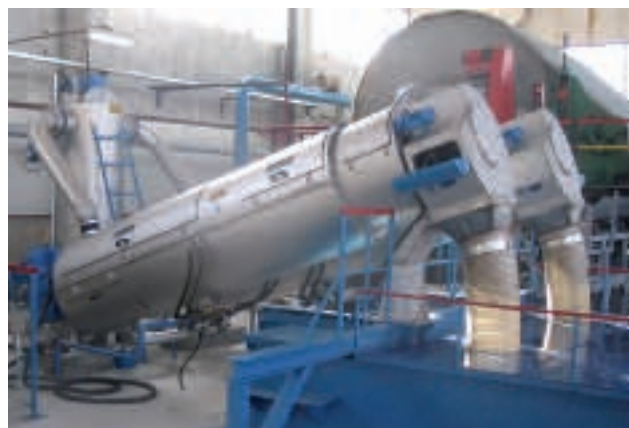
2 ROTAMAT® Screw Press RoS 3 units installed in parallel (Bulgaria)
