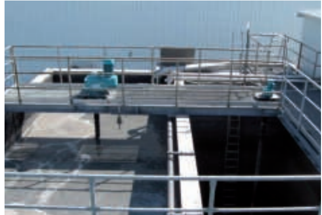
Biotank (left), mixing & balancing tank (right)
