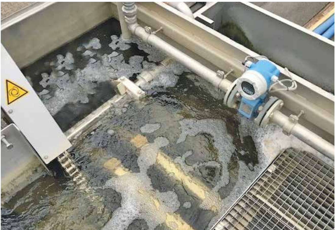
HUBER Pile Cloth Media Filter RotaFilt® in operation.
