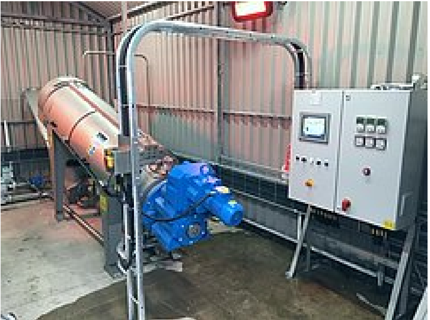
Installed HUBER Screw Press Q-PRESS@ 440.2 and Control Panel
